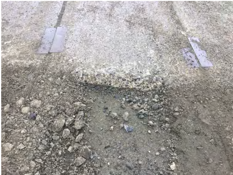
Damage to slab ends
